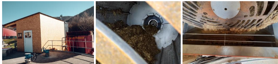
Ball mill prototype at full-scale research biogas plant "Unterer Lindenhof"
