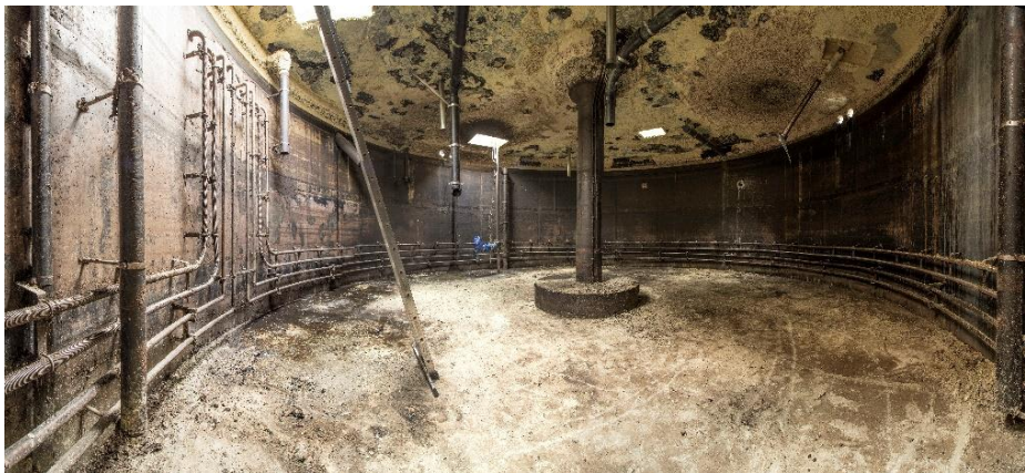
Modification measures in the fermenter of the research biogas plant for sensor-based detection of the stirring requirement (2021, University of Hohenheim)
