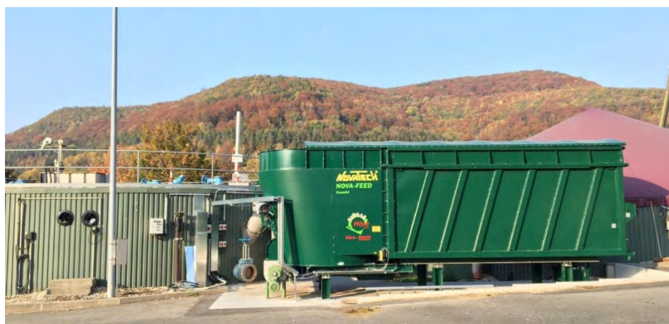
The new solid feeder at the digester 2 of the research biogas plant (Kress, 2018)
