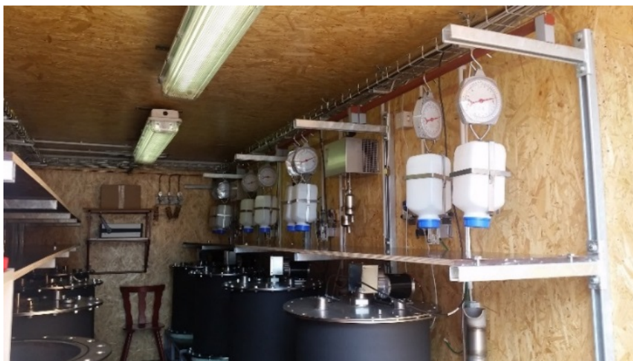
Laboratory container for hydrogen injection experiments (Lecker, 2016)
