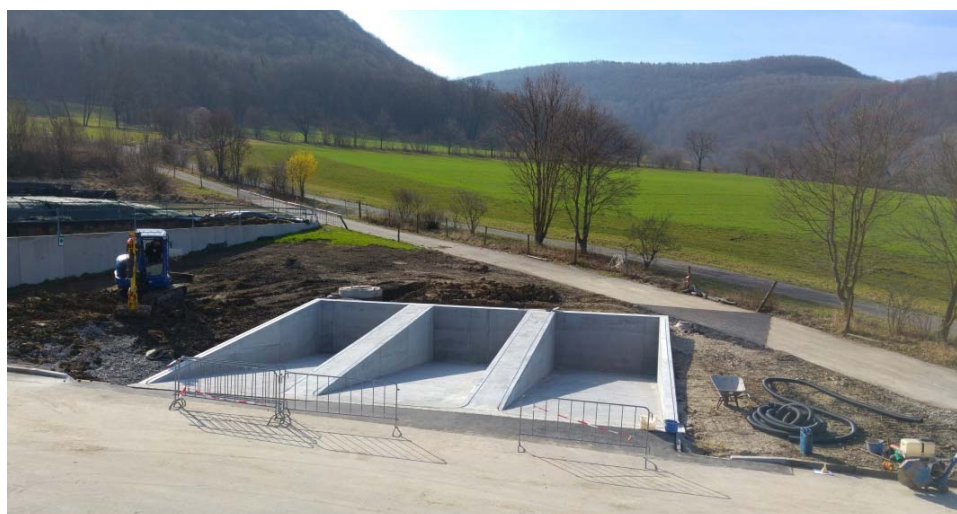
Experimental silos for sugar beet storage under construction at research station "Unterer Lindenhof"
