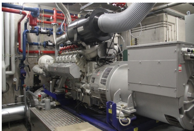
New gas CHP at the research biogas plant with an electrical output of 355 kW
