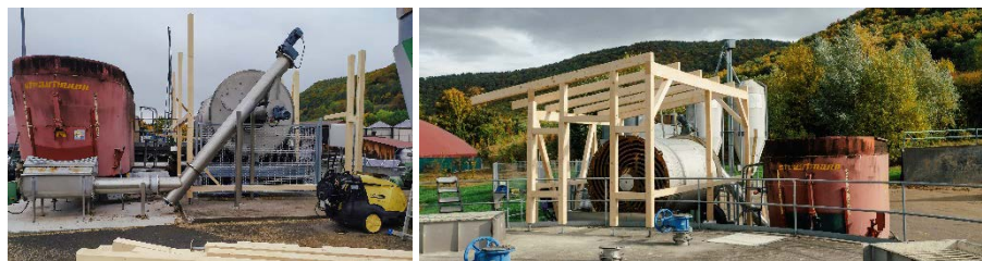
Setup and integration of the ball mill prototype at the "Unterer Lindenhof" research biogas plant
